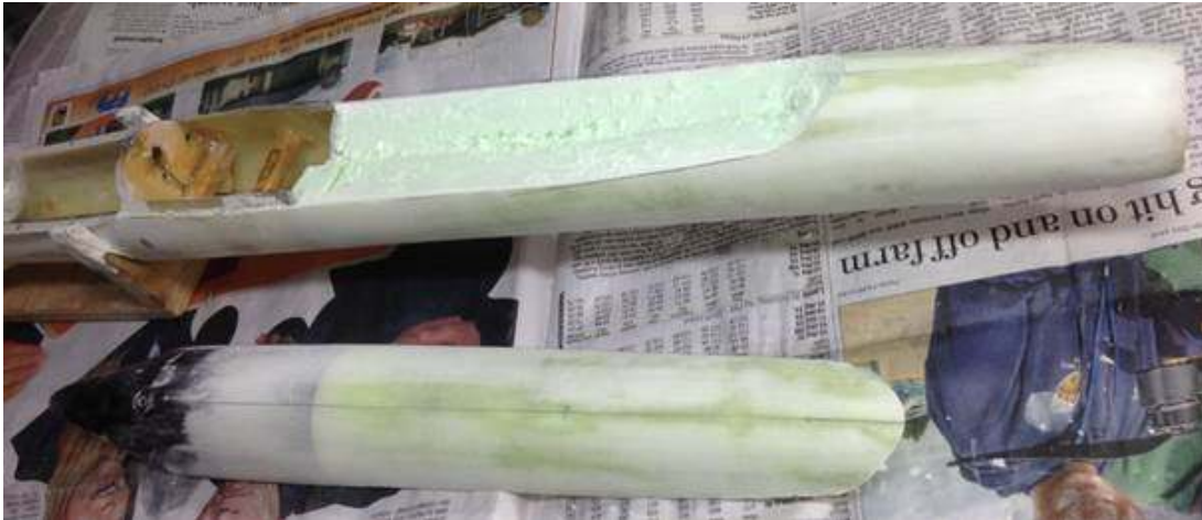
Canopy cut out ready to remove the foam to leave a new hollow front shell.
